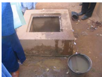
Open well and polluted water from well
